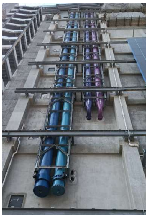
Project name: WDC01 Project location: Singapore Project type: Data Centre Project status: Completed Services: Chilled Water System Photos: Courtesy of Accesstech Engineering Pte Ltd
