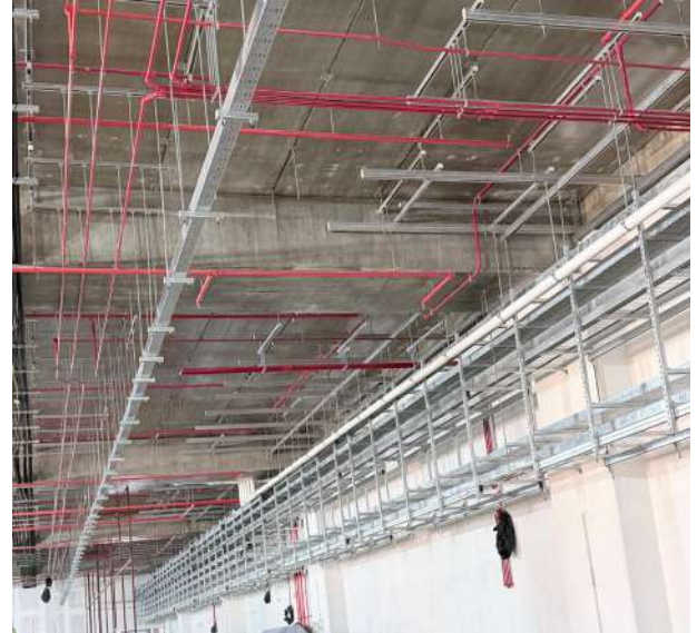
Project name: EDC01 Project location: Singapore Project type: Data Centre Project status: Ongoing Services: General Utilities Photo: Courtesy of Accesstech Engineering Pte Ltd
