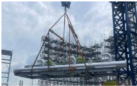
Project name: WDC01 Project location: Singapore Project type: Data Centre Project status: Completed Services: Chilled Water & Condenser Water System Photos: Courtesy of Accesstech Engineering Pte Ltd
