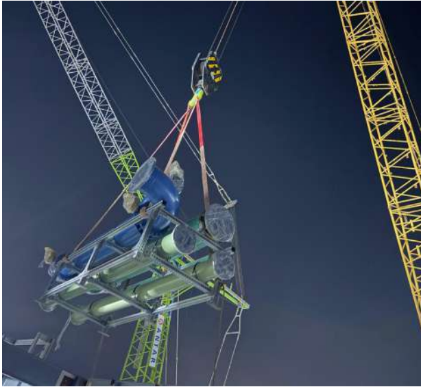
Project name: EDC01 Project location: Singapore Project type: Data Centre Project status: Ongoing Services: Chilled Water & Condenser Water System Photo: Courtesy of Accesstech Engineering Pte Ltd
